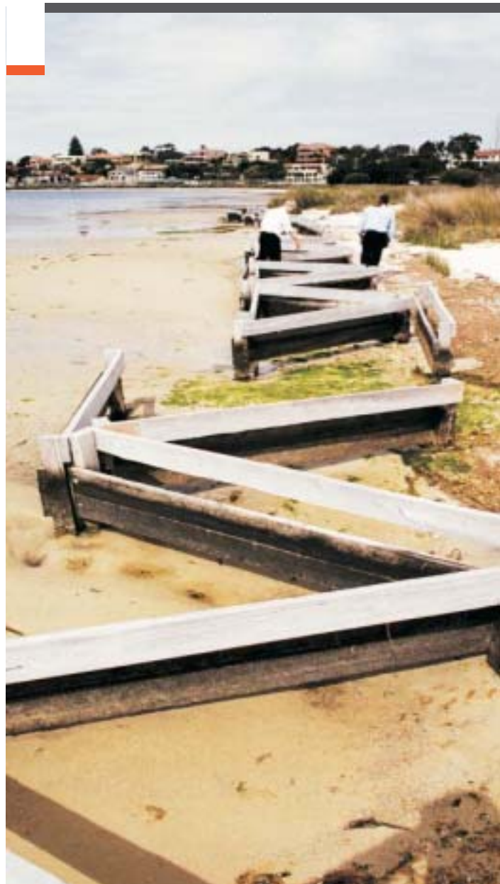
Staff reviewing the erosion barriers at our Bibra Lake, Western Australia contract
